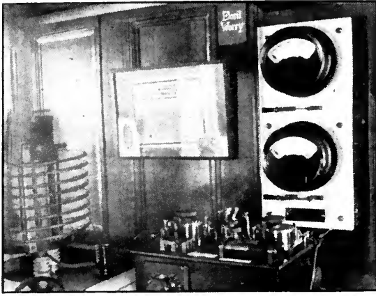
THE NEW RADIO ROOM WAS FINISHED AT LAST. And I transferred the 2 K. W. outfit to its new home. There was hardly room to get the camera in when the job was done.
